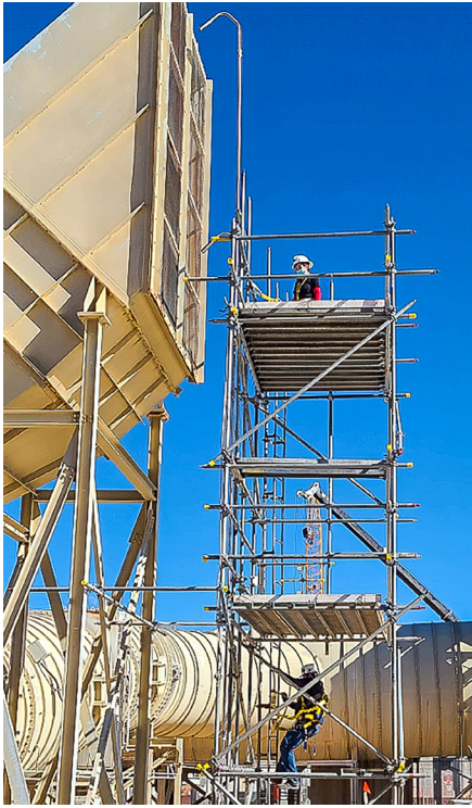
Crews on scaffolding at the exhaust face of the 700C fan, prepare for the initial bump test in January of 2021.
