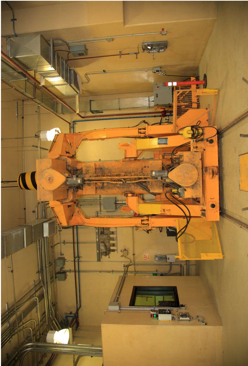
Figure B4-11 Facility Cask Loading Room and Facility Cask Rotating Device
