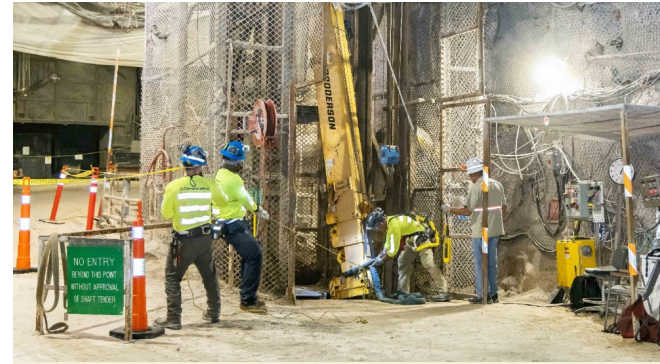
Work begins in the WIPP underground to refurbish the salt loading pocket infrastructure
