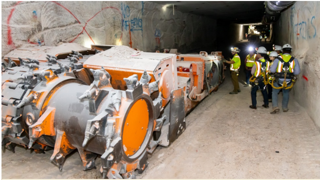
An underground continuous mining machine prepares to mine salt at the new utility shaft
