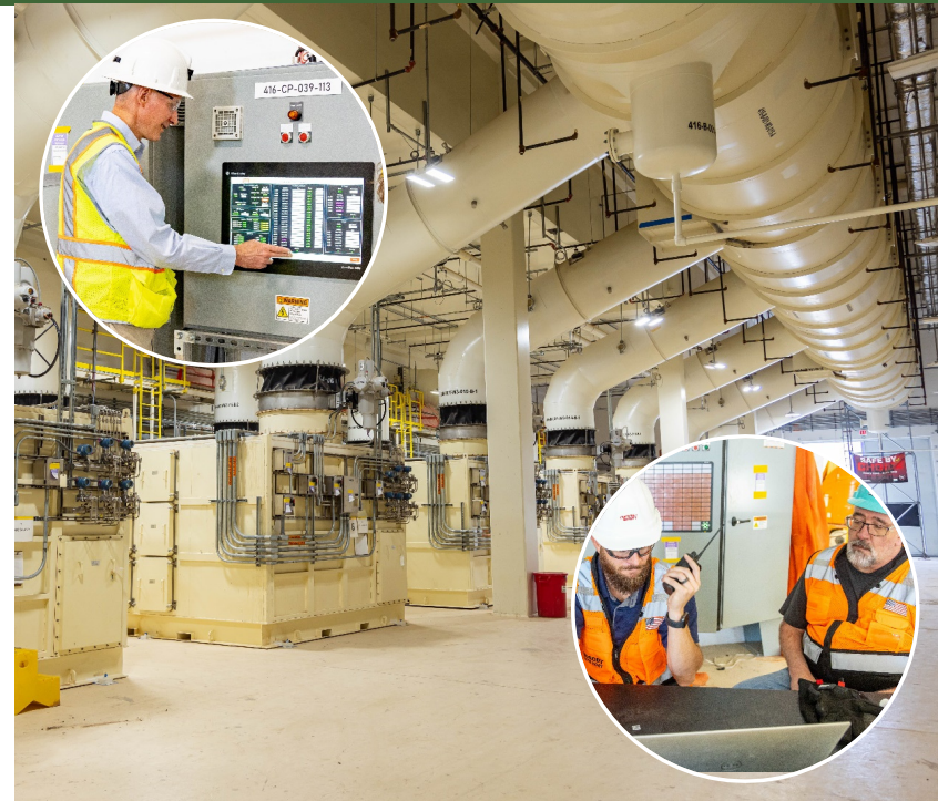
Above: Filter banks inside the SSCVS New Filter Building Inserts: Filter fan control panel (above), systems testing (below)
