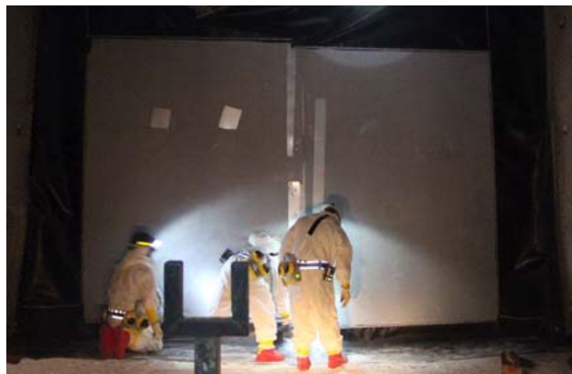
WIPP workers install rubber flashing around the metal bulkhead recently installed in Panel 6.
