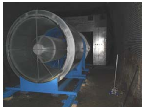
SVS installed in the WIPP underground.
