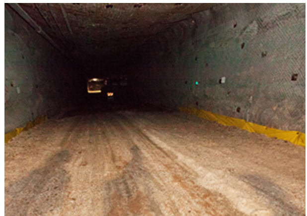
Brattice cloth placed on the floor of the repository and covered with run of mine salt
