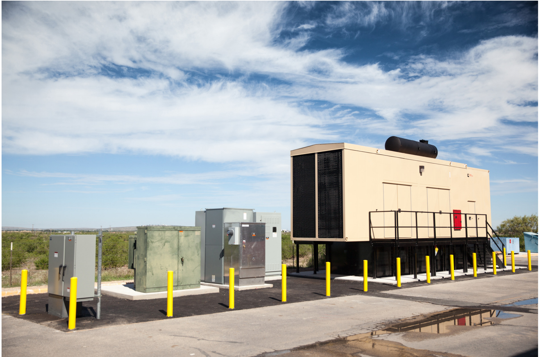
Skeen-Whitlock Building Emergency Operations Center Backup Diesel Generator
