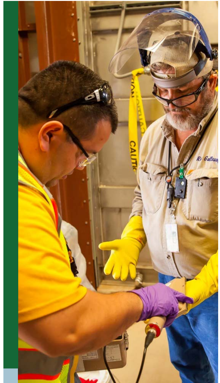
Workers complete a HEPA filter change in the filter building
