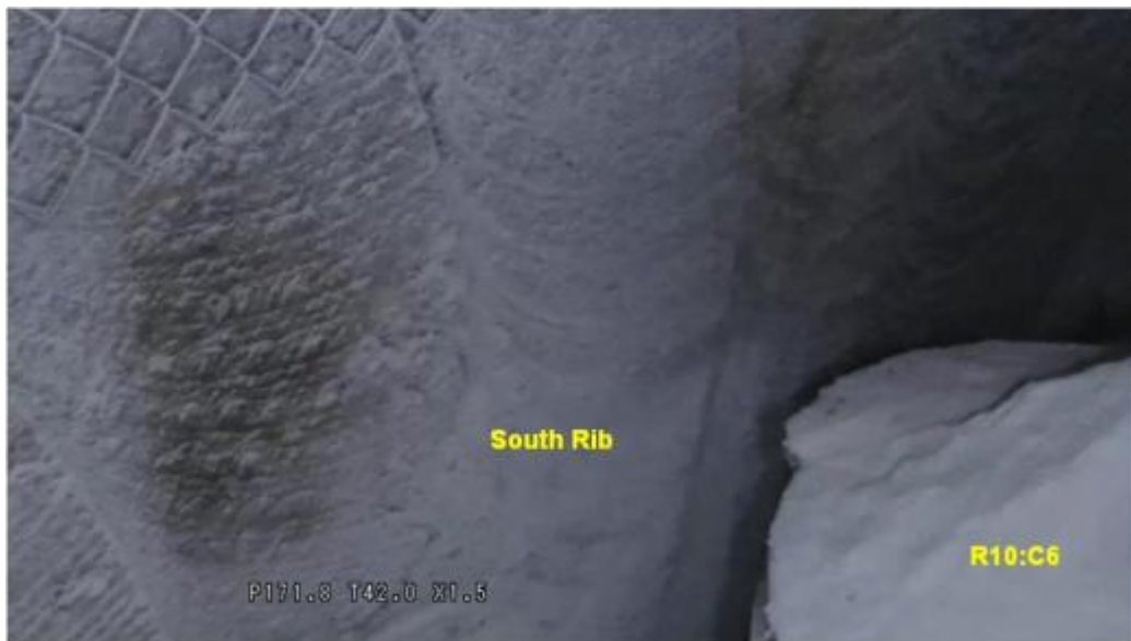
Figure 6-28: Flame Impingement Evidence on South Rib near Row 10
