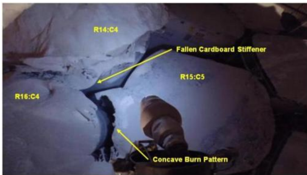
Figure 6-6: Evidence of Flaming Combustion Irregular Edge Surfaces at R15:C5
