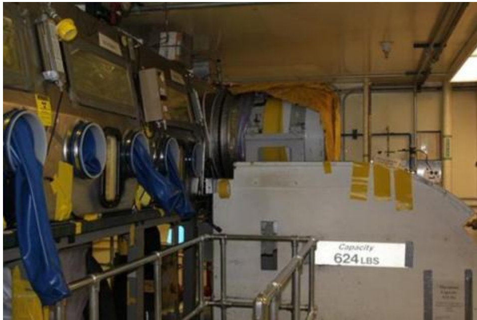
Figure ES-3: Waste Characterization Glovebox in WCRRF at LANL
