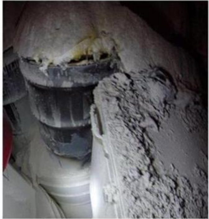
Figure 2-3: Drum 68860 Lid Failure
